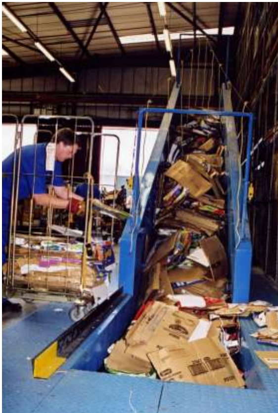
The Co-op Fareham depot prefers the narrow conveyor we installed here as it takes up so little room. It feeds our LP50HM horizontal baler. Note the double emergency stop ropes every two metres.
