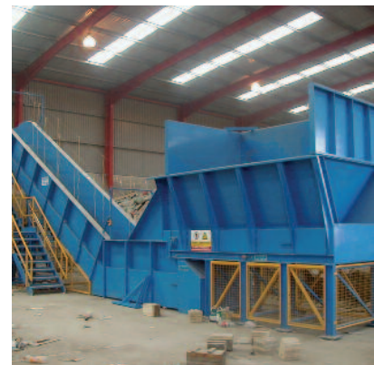
Inclined chain conveyor with feed hopper, feeding metered load to sorting cabin
