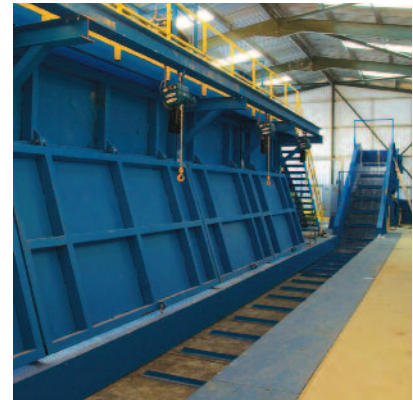
In-floor chain conveyor with rubber belt and flights at May Gurney
